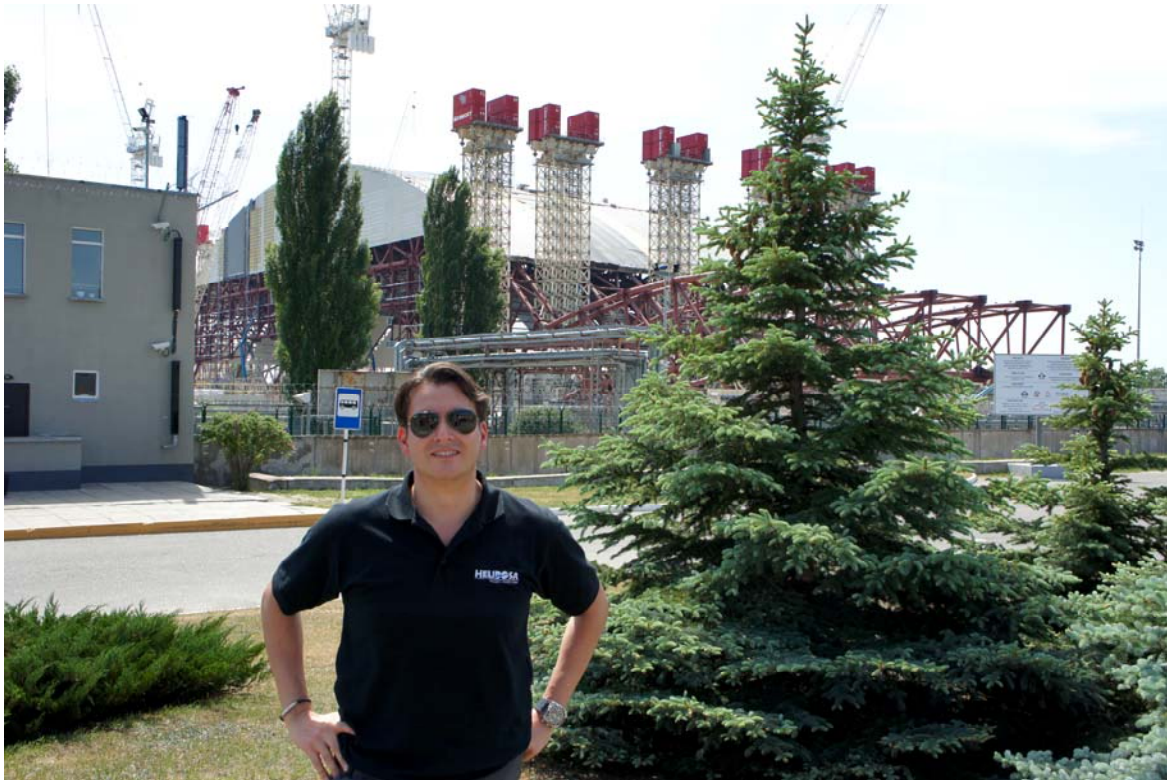
(Above) A.C. Frieden stands near the new sarcophagus that is still under construction. The new structure is intended to replace the damaged reactor's current containment.
