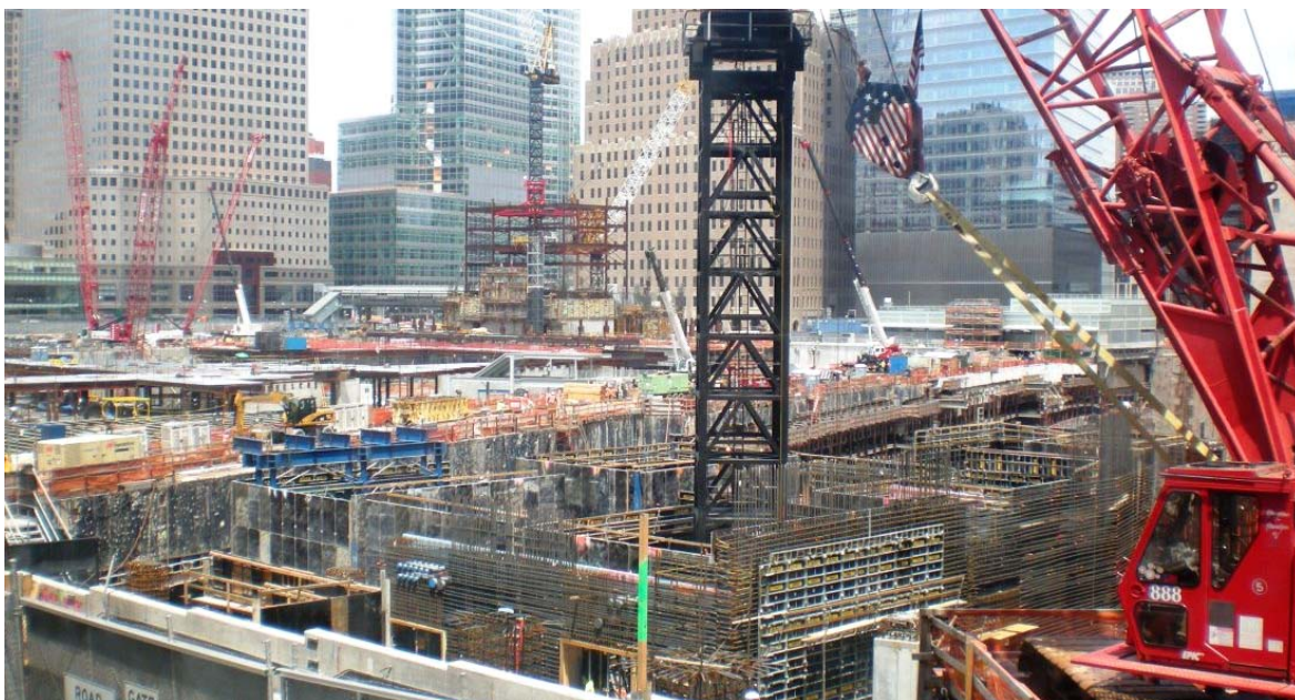
Photo above: View of the construction at "Ground Zero", the site of the former World Trade Center that was destroyed on September 11, 2001.
